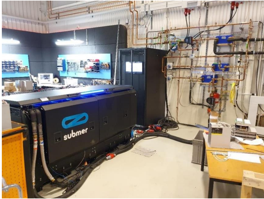
Figure 2. Submer SmartPod to the left and Liquid cooling testbed (LCT) to the right at RISE ICE T&D.
